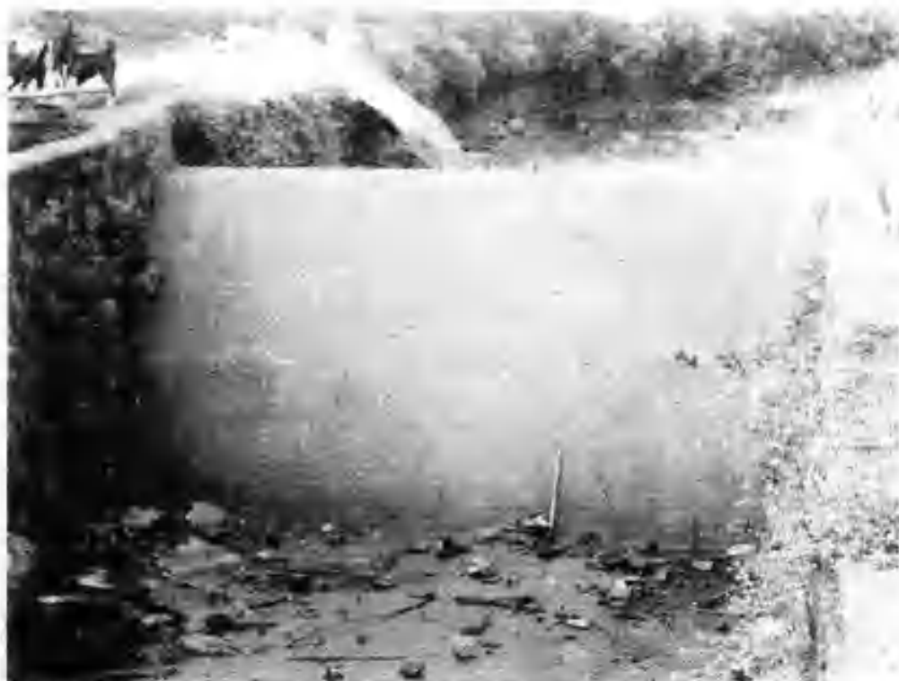
Photograph of Check Dam and Settling Tank
