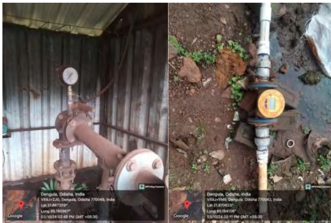
Figure 7.12 : Flow meter installed in groundwater withdrawal wells
