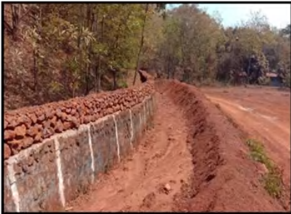
Fig 7.2: Retaining Walls and Garland Drain in Mining area
