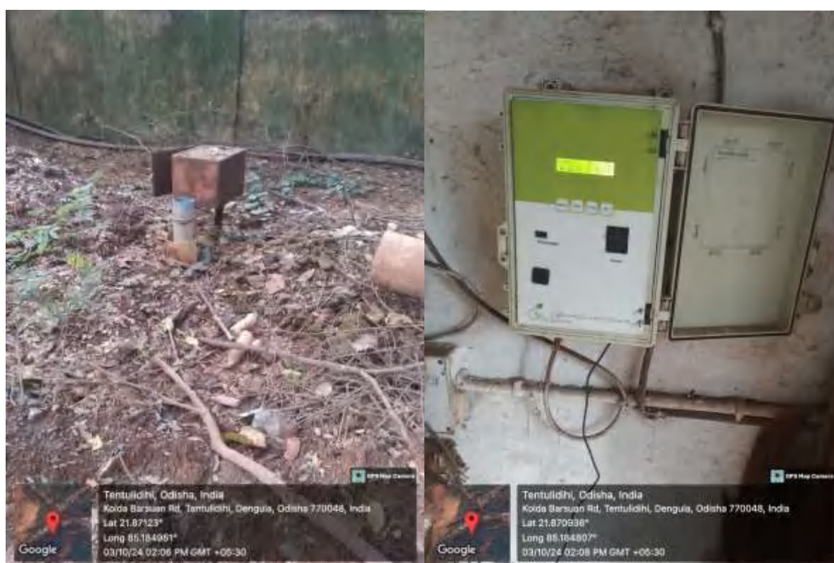
Figure 7.1: Piezometer well with DWLR within the lease area.
