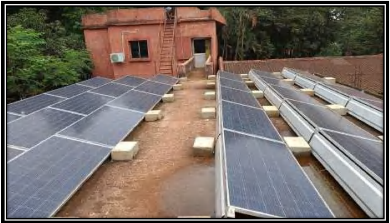
PHOTOGRAPH SHOWING 30KVA SOLAR POWER
